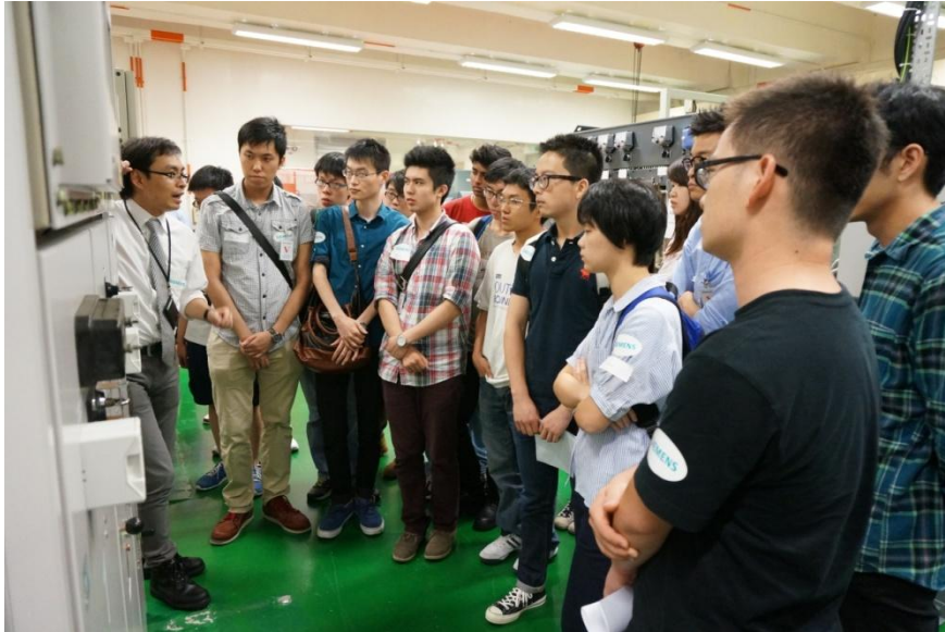
Experienced engineers from Siemens introduced the company's switchgears which are currently operated in our customer's power substations.
